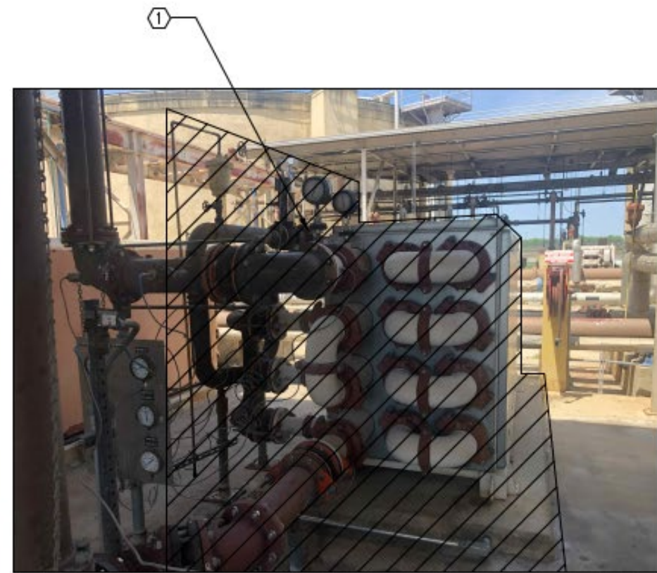
DESCRIPTION: TYPICAL FRONT VIEW OF HEAT EXCHANGER HIGHLIGHTING THE SLUDGE AND HOT WATER INLET AND OUTLET CONNECTIONS.
