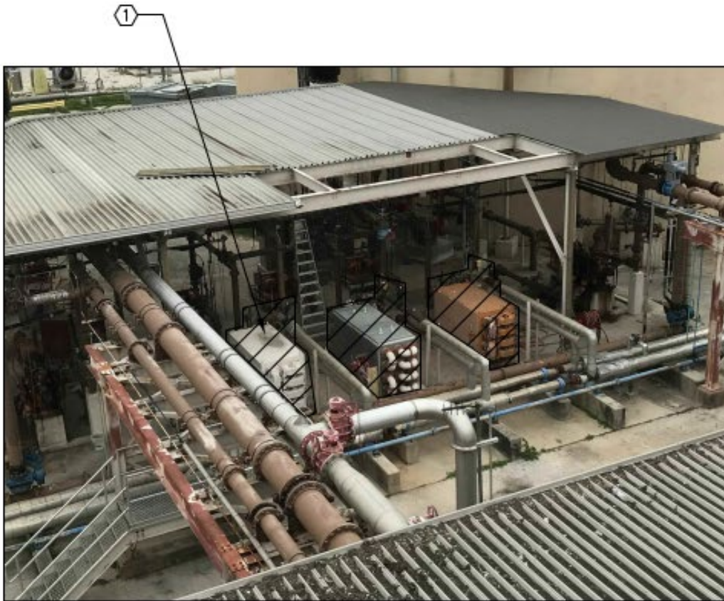
DESCRIPTION: AERIAL VIEW OF PUMP STATION NO. 3 HIGHLIGHTING ALL THREE HEAT EXCHANGERS. PUMP STATION NO. 4 IS TYPICAL OF PUMP STATION NO. 3 HOWEVER THE LAYOUT IS MIRRORED.
