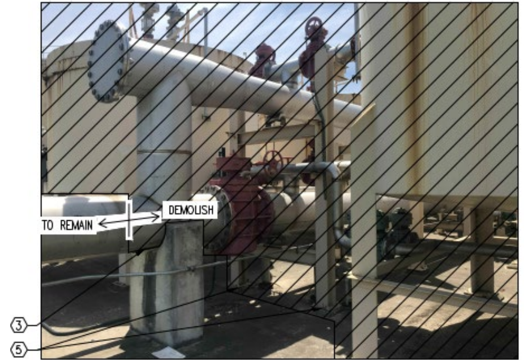
DESCRIPTION: VIEW OF IRON SPONGE PIPING FACE WEST. THE HEADER SHOWN RUNS WEST TO THE GAS FLARE STATION.
