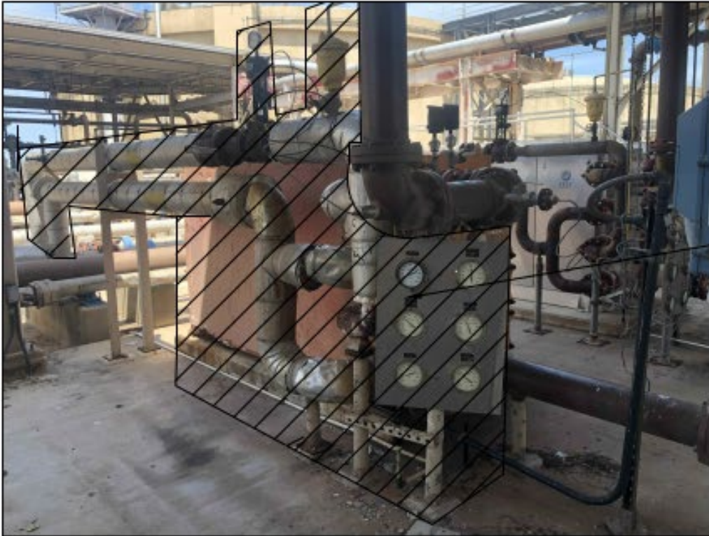
DESCRIPTION: TYPICAL SIDE VIEW OF HEAT EXCHANGER HIGHLIGHTING HOT WATER PIPING AND EQUIPMENT AS WELL AS GENERAL INSTRUMENTS.
