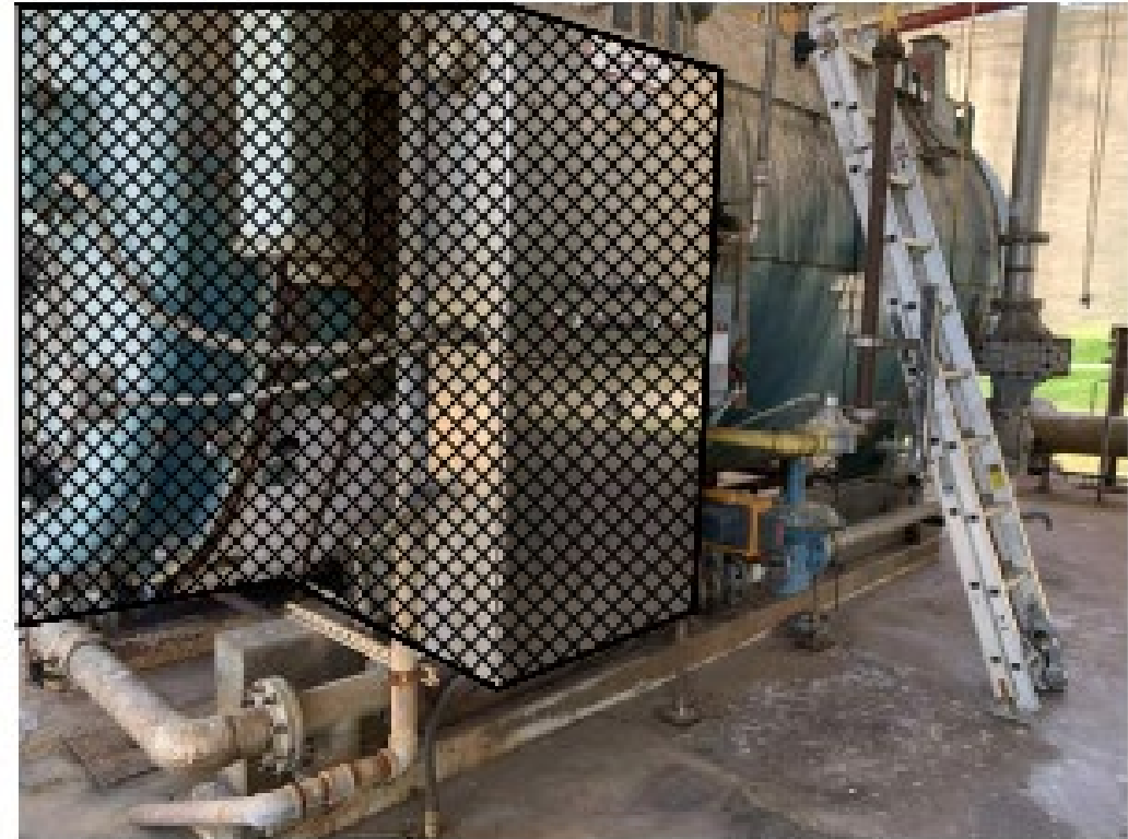
DESCRIPTION: BOILER #1 CONTROL PANEL
