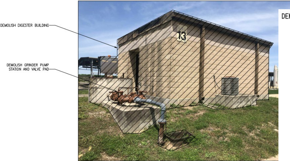
DESCRIPTION: VIEW OF SOUTH SIDE OF DIGESTER BUILDING, GRINDER PUMP STATION, AND VALVE PAD.
