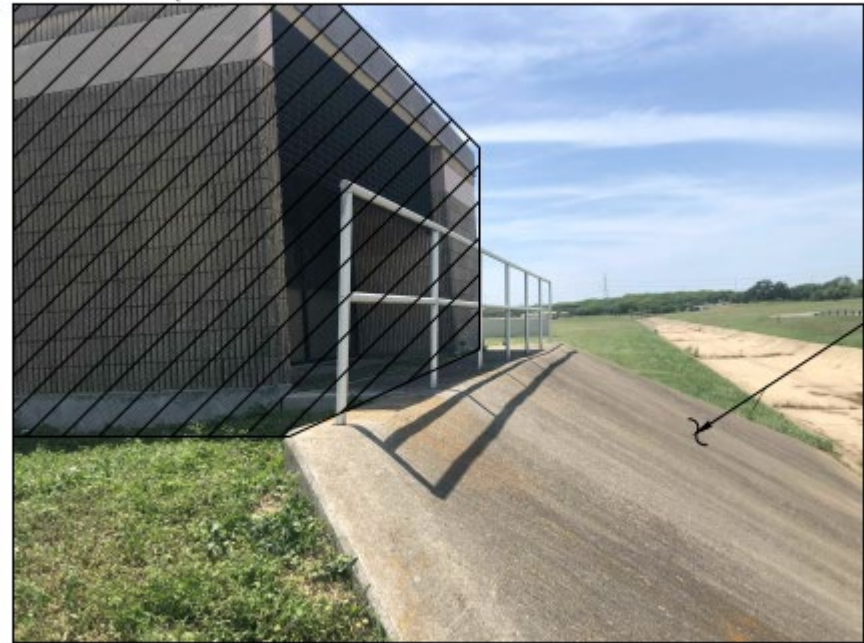
DESCRIPTION: VIEW OF NORTH SIDE OF DIGESTER BUILDING AND CONCRETE RETAINING WALL FACING WEST.
